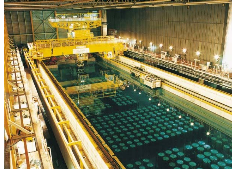
Used Fuel Storage Pond at Sellafield (UK)
