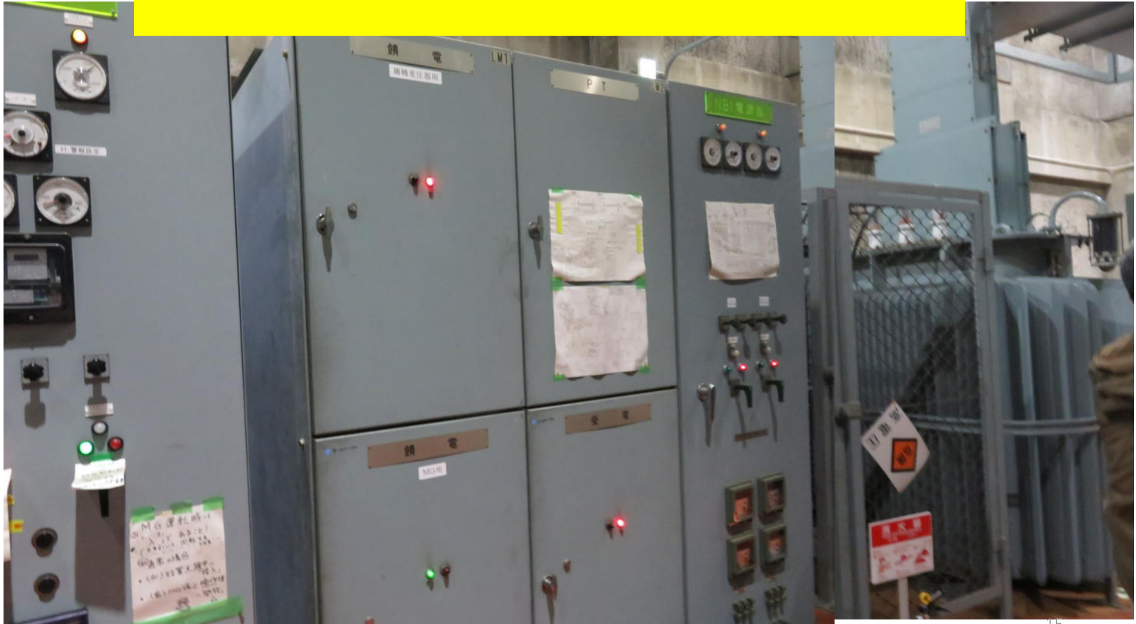
Rows of power control panels for electric generators and NBI equipment
