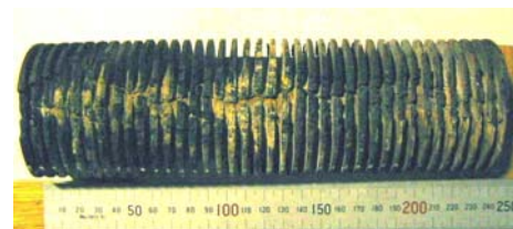
Fig. 5 Example of physical burnout of boiler tube.
