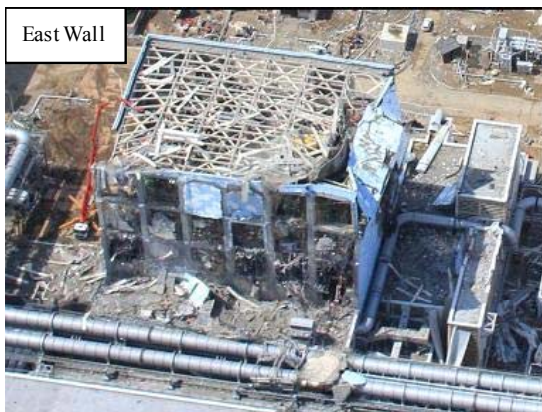
Fig.21 Appearance of Unit 4 R/B after explosion.
