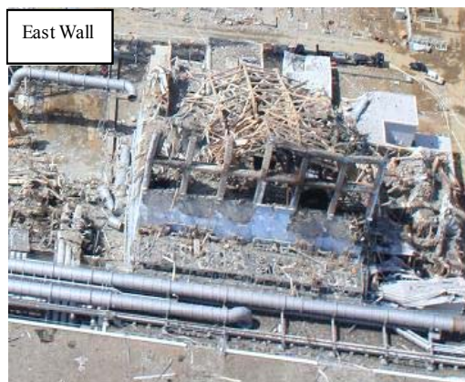
Fig.19 Appearance of Unit 3 R/B after explosion.
