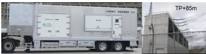
(a) 4000 kVA mobile gas-turbine generator at 31 m parking and GIS at 85 m height (Hepco).
