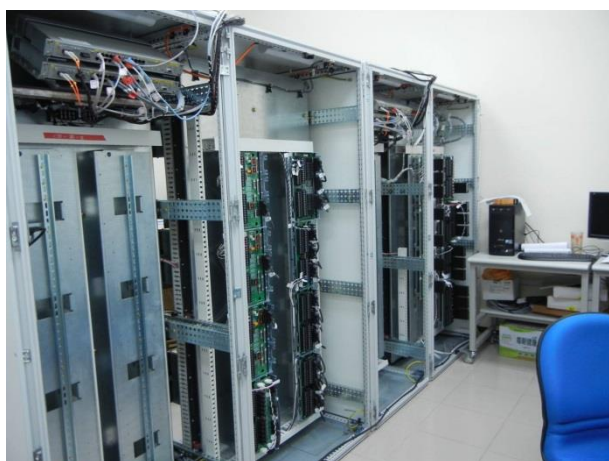
Fig.4 Physical view of FSES based digital system validation test platform – 2.
