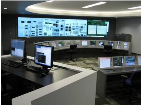
Fig.2 US-APWR V&V facility.
