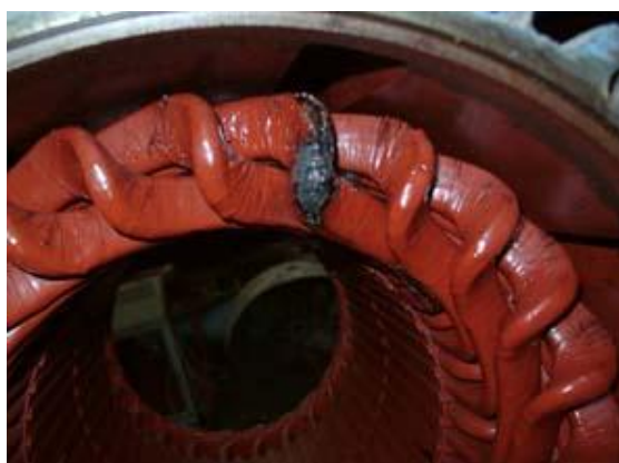
Photo 3 Insulation deterioration of coil winding.
