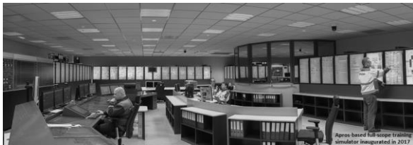
Fig.5 The control room of the new full scope training simulator of Loviisa.
