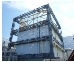
(b) Steel structure for containment cover of explosion-ravaged reactor building was built. (Unit 1)
