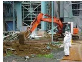
(d) Removal of debris contaminated and scattered by explosion is in progress to reduce the air dose rate. (Unit 4)
